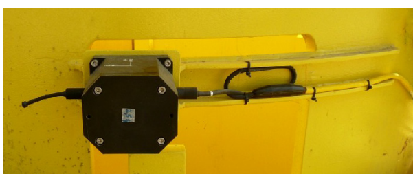
Figure 9.9 Example of proper cable routing
