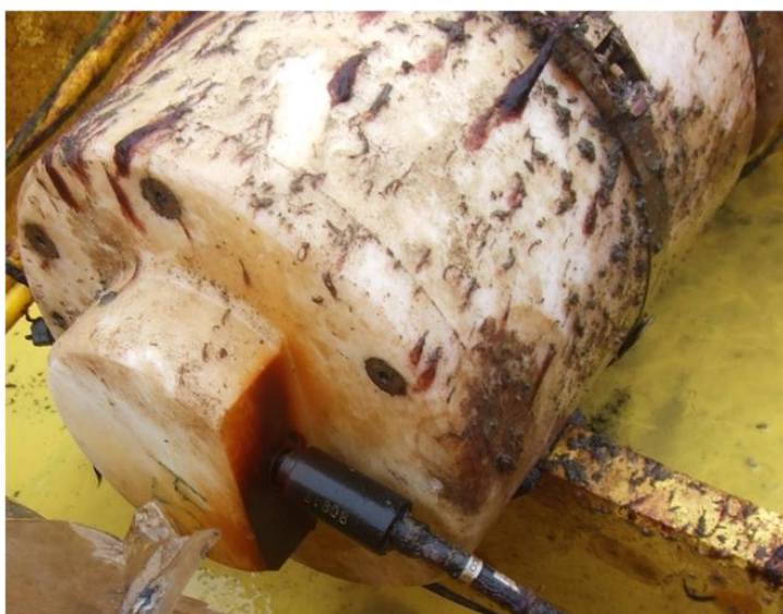
Figure 10.3 Burnt and galvanic corroded connector caused by stray currents in the water probably originating from a broken cable isolation
