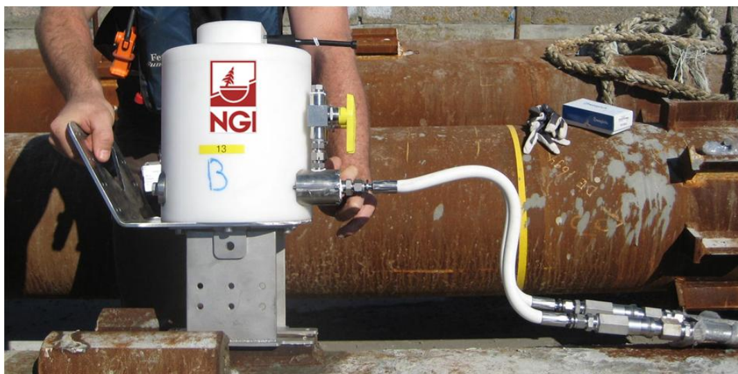
Figure 3.30 Trial fit of seabed sensor head containing two differential pressure sensors serving to hydraulic piezometer lines which are hooked up by the (white) flexible jumper hoses. This unit is equipped with manual operated bypass valves to sea (yellow handle).
