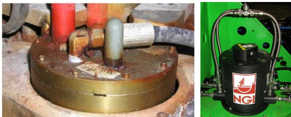
Figure 7.1 Galvanic corrosion on metal enclosure with connectors in different metal grade (left). “Corrosion safe” synthetic enclosure in Delrin for shallow water with connectors/outfitting in stainless steel (right)
